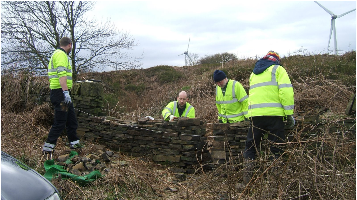
One of the recent but now regular volunteers David M passed on his knowledge of repairing dry stone walls, to repair 5 year old damage to the boundary wall from an old car accident leaving access gap for walkers and wildlife.
